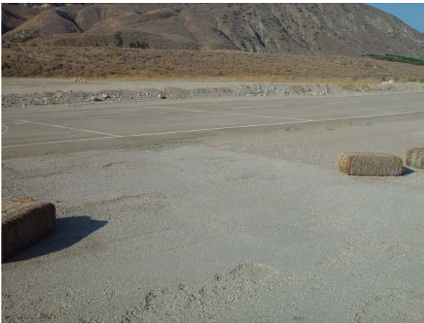
Freshly “excavated” taxi area—The damage is not yet fixed.
