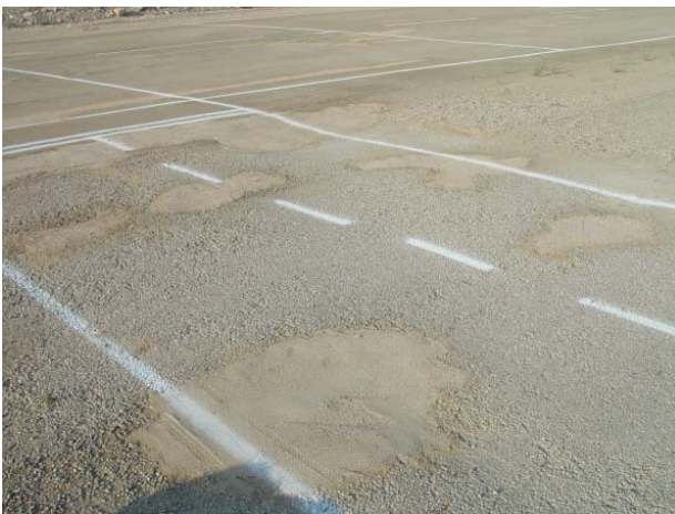
The same taxi area after applying the polymer patches and re-striping the runway markings
