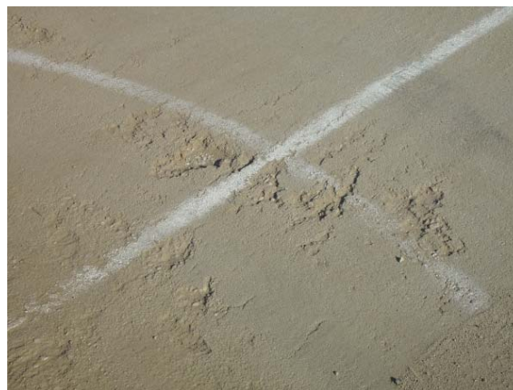
Detail of the damage before it was fixed
